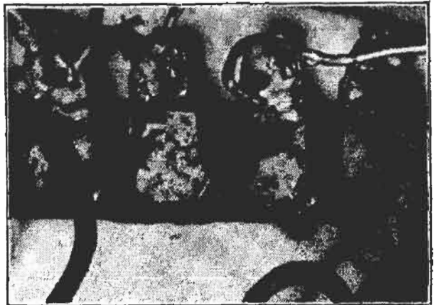
An example of poor soldering. The lumpy, cracked appearance shows too much solder was used and the joints were not heated enough.
